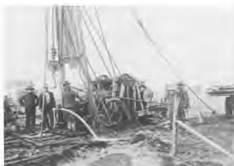
A private drilling crew has just completed construction of an artesian well with a cable tool rig.
