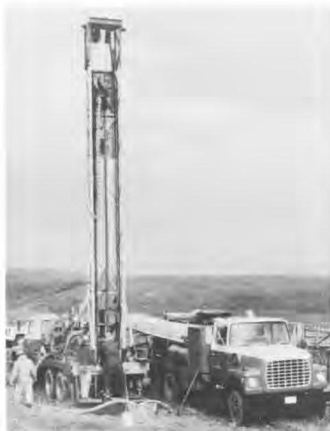
Survey drill crew using a rotary drill rig for test drilling during a county-wide investigation.
