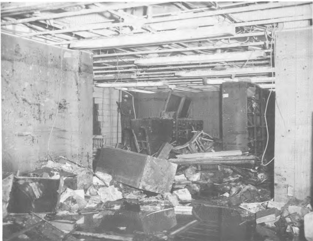
Office area after flood.
