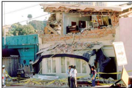
Top, Fire in San Francisco, California, after 1989 Loma Prieta (World Series) earthquake. Bottom , Damage to unreinforced masonry building from 1994 Northridge California, earthquake. Photos courtesy Karl V. Steinbrugge Collection, University of California, Berkeley, Earthquake Engineering Research Center.
